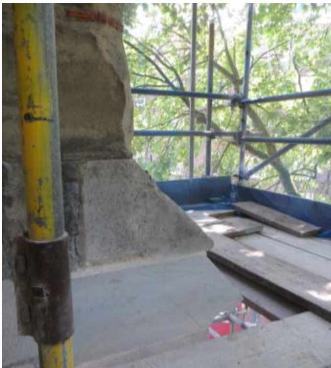
Figure 4: Replacement stone with weathering detail to buttress
