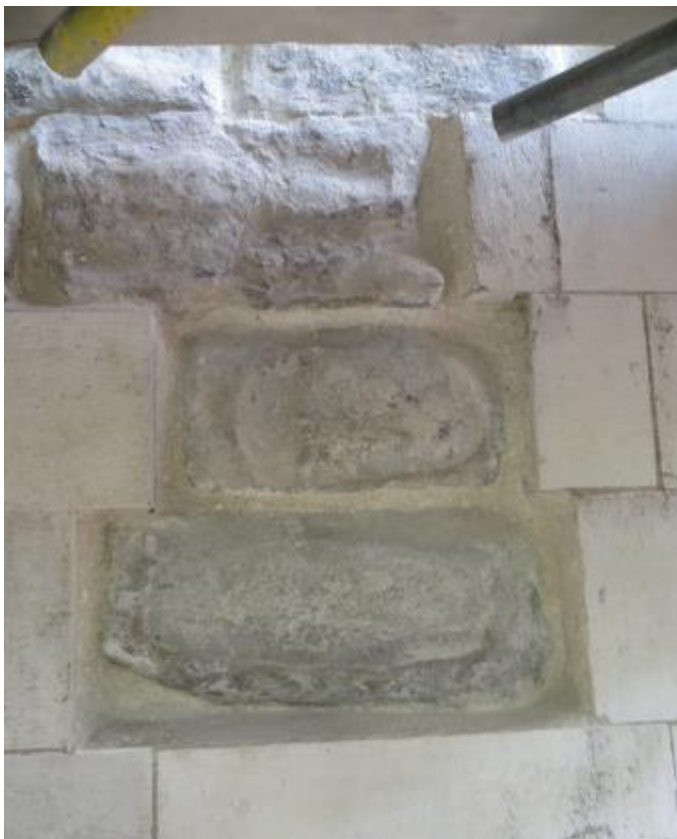
Figure 7: Light clean of Kentish ragstone to remove sulphate crust, remove cement pointing and point with lime mortar where necessary. This will enable the building to evaporate moisture externally.
