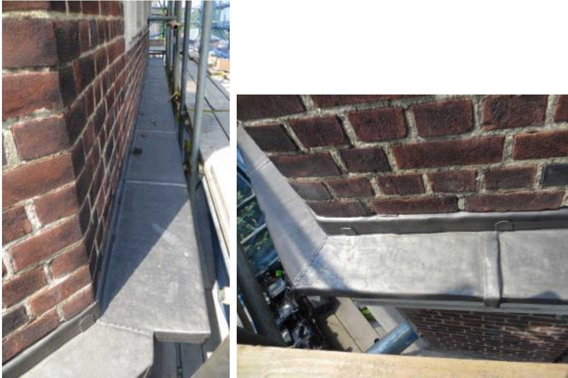
Figure 2: Renewal and width extension of moulding with lead flashing to throw water away from the tower. Lead work carried out to BS 6915:2001
