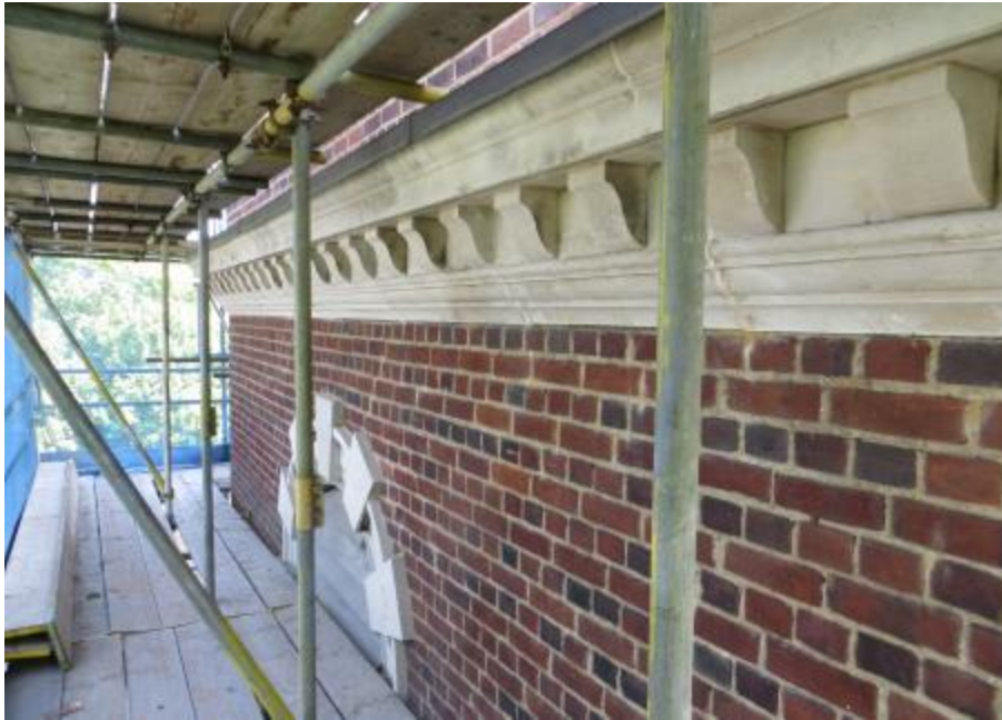
Figure 3: Soot cleaned from cornice and renewed lead flashing done to BS 6916:2001. Repointing of open joints in brick work with lime mortar. Beeswax on window louvres to shed water.
